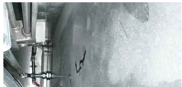
View inside an exhaust plenum fitted with UV-C lamps after several weeks of use
